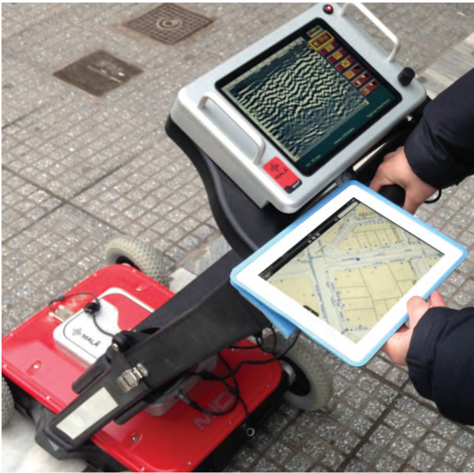
↑ Aided by mobile GIS, an EYATH employee uses a ground-penetrating radar device to more accurately identify underground network assets.
